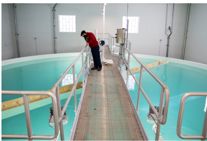
Michael Crawford, the Collinsville water plant's chief operator, inspects a clarifier tank at the facility on Feb. 11. The Metro East town is one where contains levels of PFAS that exceed state and federal standards. E. JASON WAMBSGANS/CHICAGO TRIBUNE
